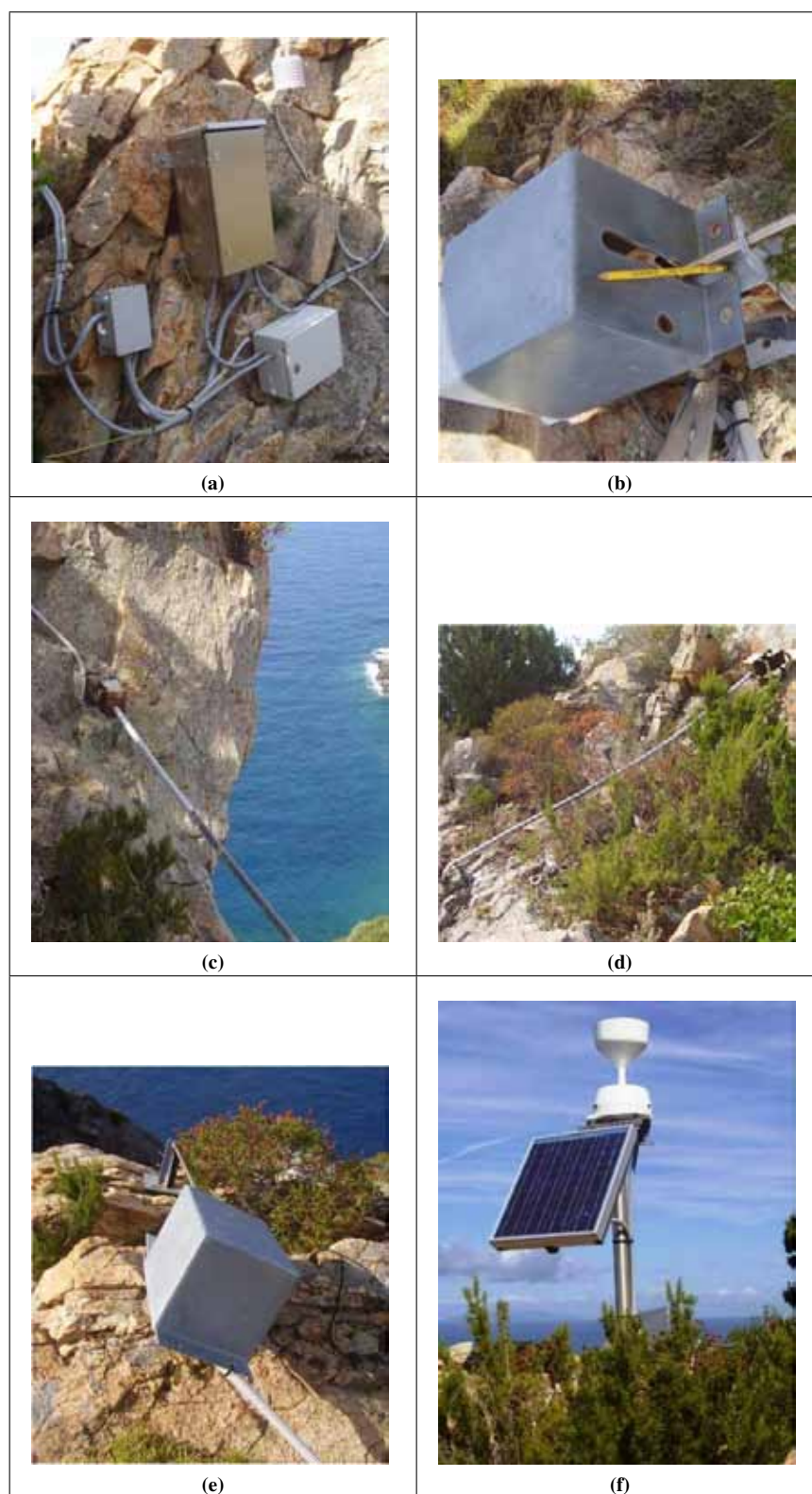
Figure 7.32: Pictures of the components of the Monitoring system installed at Punta del Timone, Elba Island (May, 2010). a) Datalogger and Gateway b) Extensimeter E3 c) Extensimeter E1. d) Extensimeter E2 e) Extensimeter E4 f) Pluviometer.
