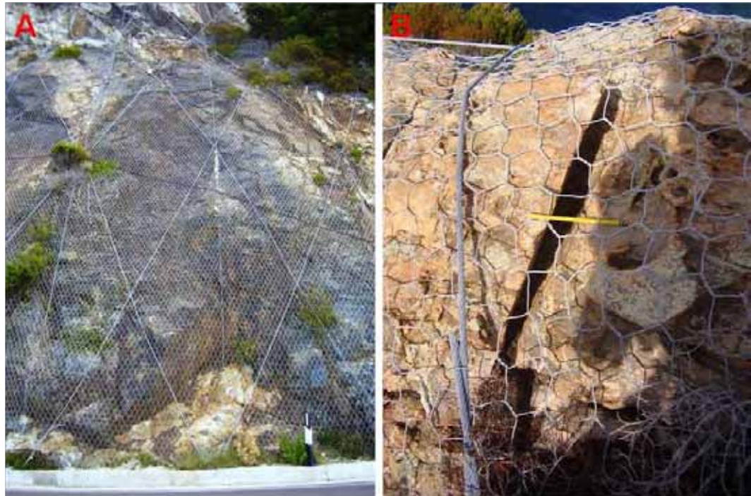
Figure 7.15: Pretensioned boulder net with hexagonal mesh installed in the intervention of '99-'01 (April, 2010).
