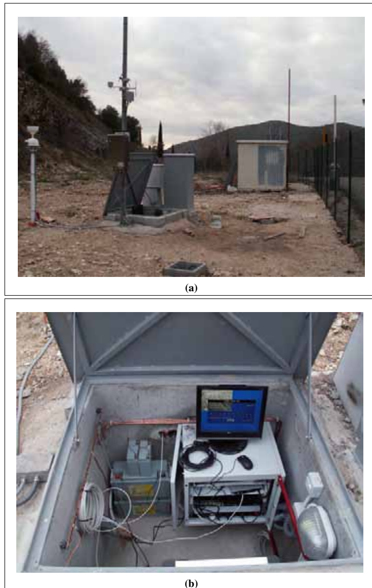
Figure 6.4: The shelter contains the gateway, batteries, and central recording unit. a) View of the shelter from west. b) Inside view of the shelter (February, 2010).
