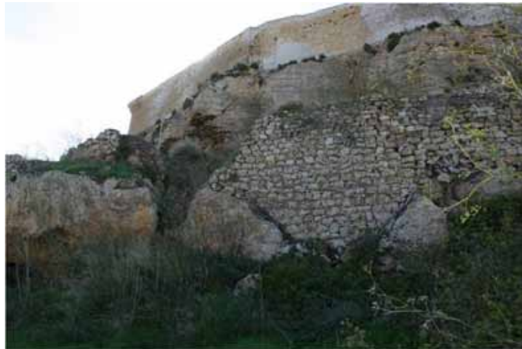
Figure 5.24: Abandoned terrace protecting walls partially built on rockfall debris (May, 2010) .
