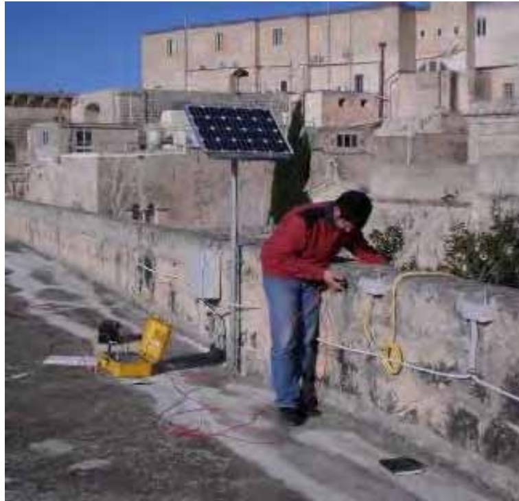
Figure 4.44: Solar panel to provide the RAU power supply (taken from [5]).
