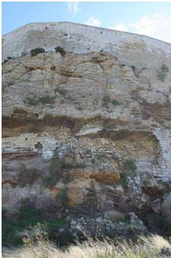
Figure 5.12: Degraded and partially collapsed underwalling masonry (April 2009).
