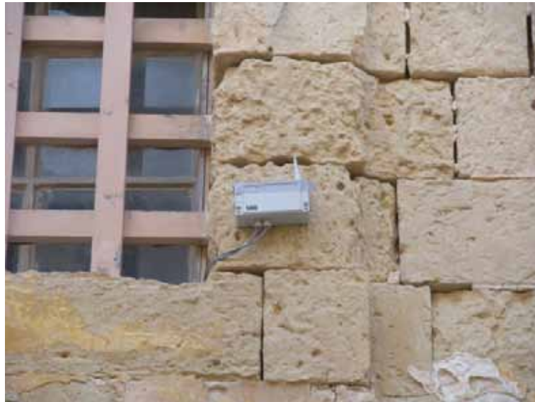
Figure 4.42: Local Transmitter Unit (LTU) (November, 2010).
