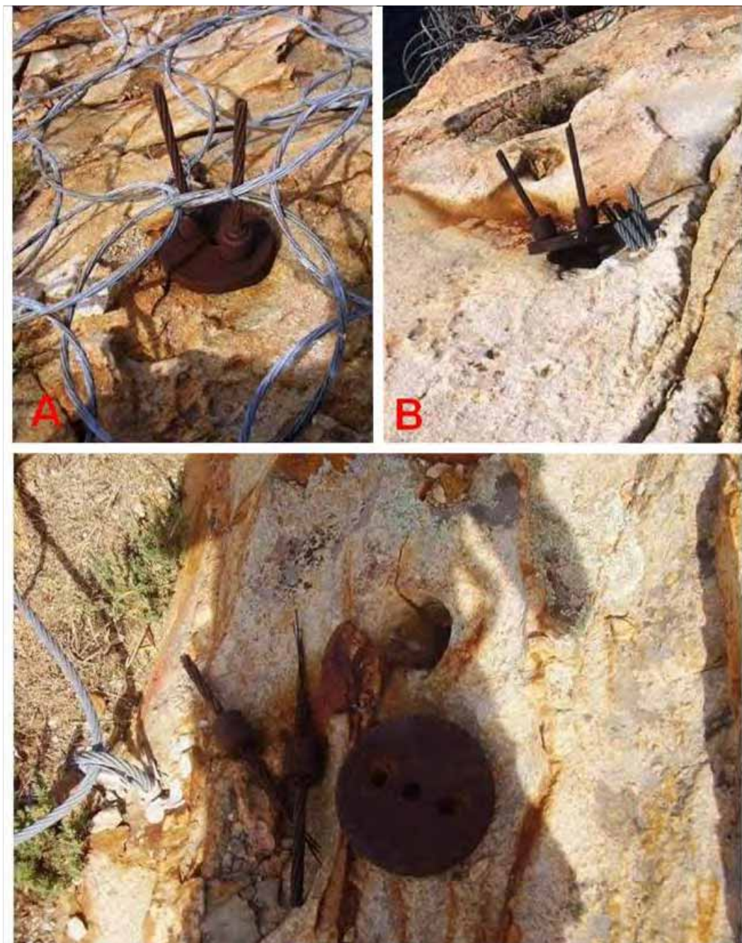
Figure 7.10: Tie-in mounted during two-year '88-'89 A-B-C); broken rods (April, 2010).
