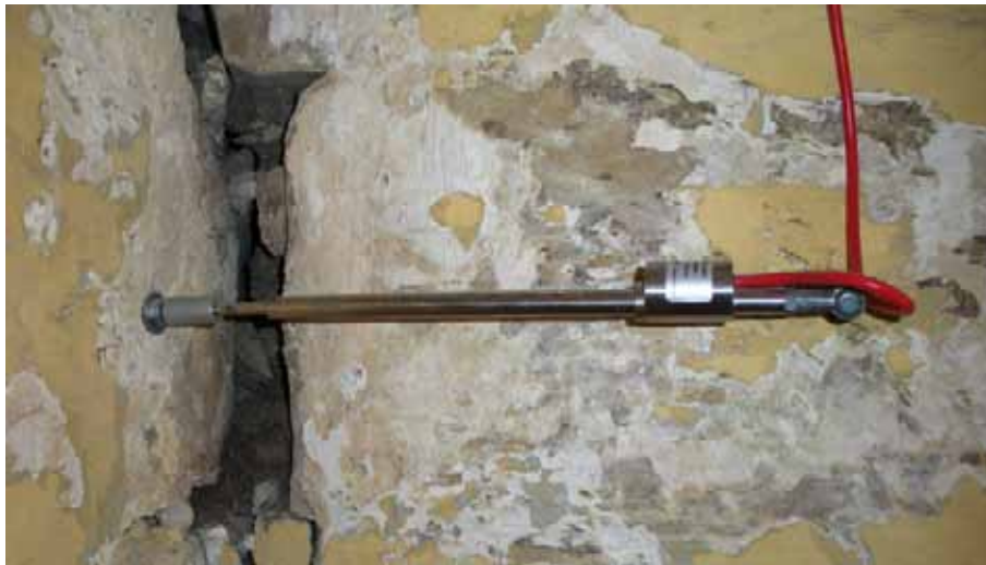
Figure 4.36: Crack gauge installed on a wall of Mdina, Area C..
