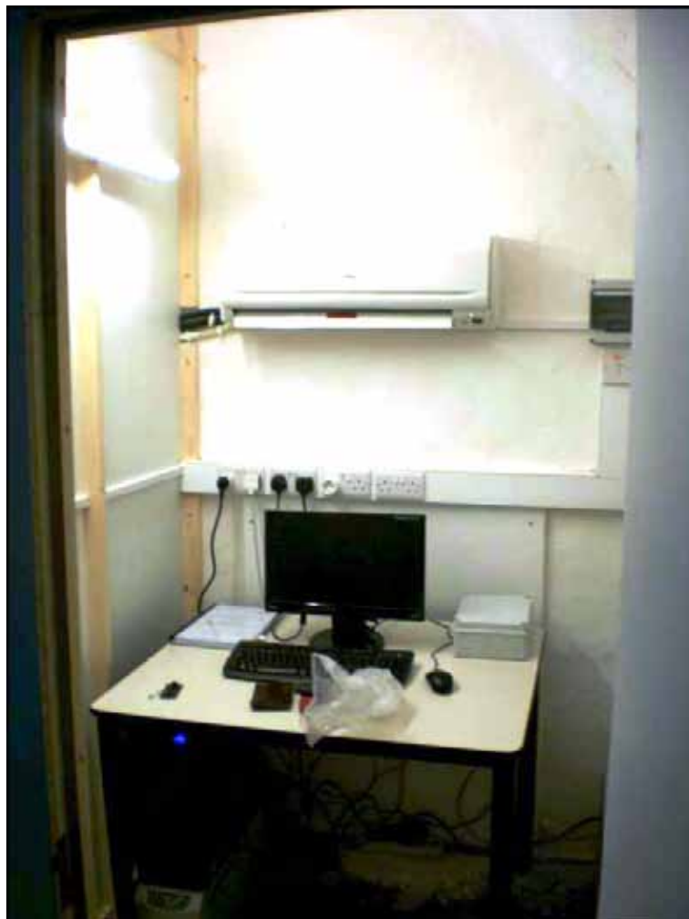
Figure 4.43: Server Room located inside the tower of the standard (March, 2010).
