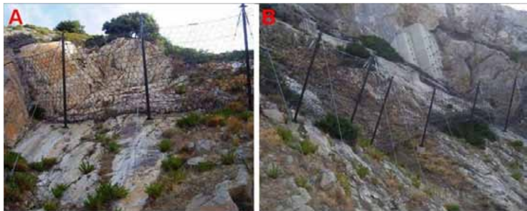
Figure 7.16: Rockfall barriers relating to the intervention of the '09-'10 (April, 2010).
