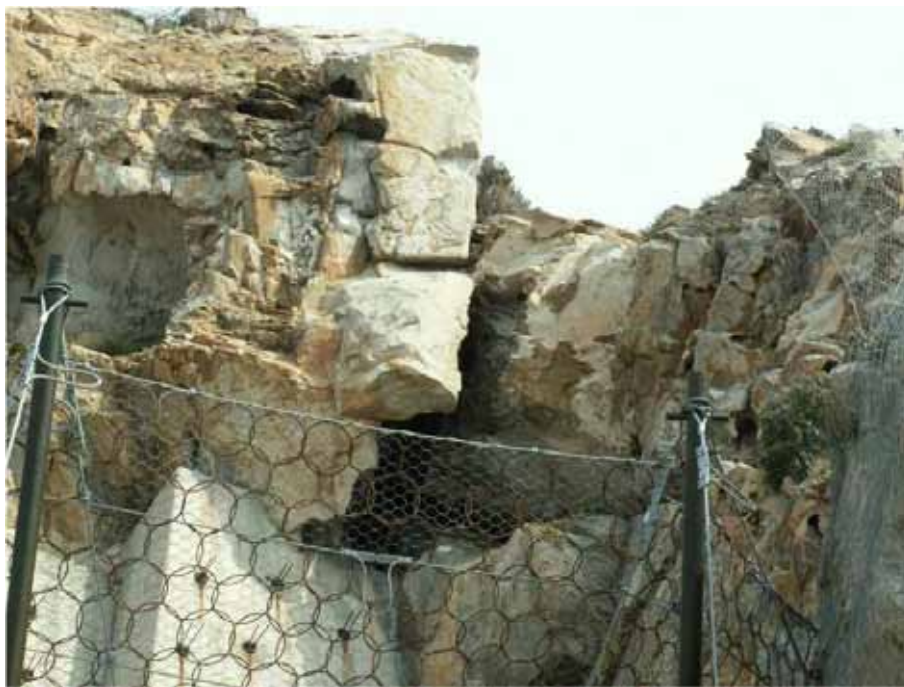
Figure 7.17: View of an unstable block within a located in the central portion of the rock mass 3 (May, 2010).
